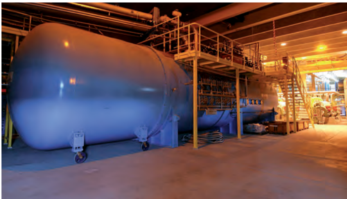
One of the eight, 18 kW cold-boxes at 4.5 K, used in the LHC.
