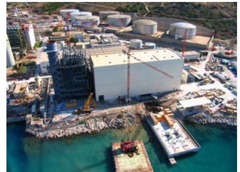
Lavrion Combined Cycle (Greece) 109 FA-GE 400 MWe
